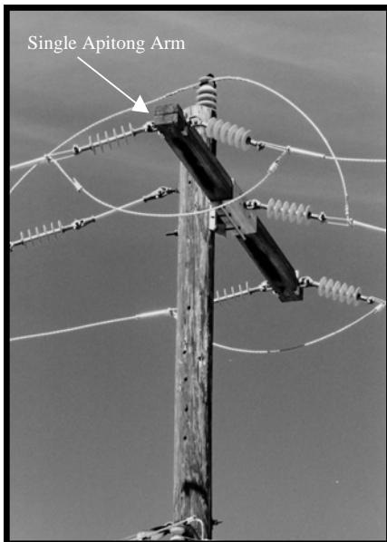
Photo 3 Distribution Pole Employing a Single Apitong Wood Crossarm with Jumpers under the Arm to Prevent Nesting and Electrocutions
