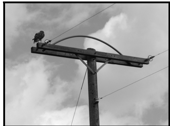
Photo 5 PVC Homemade Stick Deflector at a Double Deadend Structure
