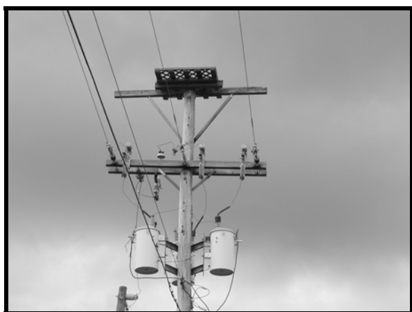
Photo 6 Elevated Nesting Platform on a Partially Unprotected Structure
