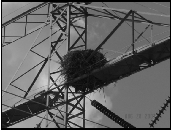
Photo 1 Golden Eagle Nest to be Relocated Due to Streamer Issues on V-String Insulators
