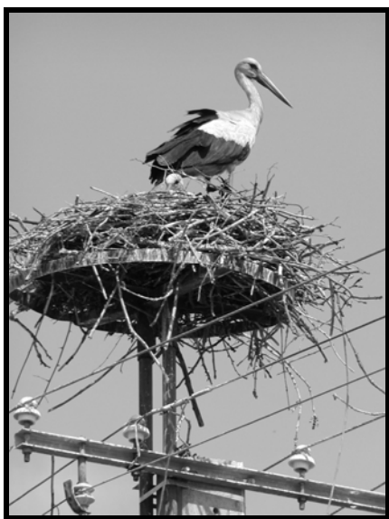
Photo 7 Power Poles with Elevated Nests should be Retrofitted to Prevent Electrocution of Young Birds
